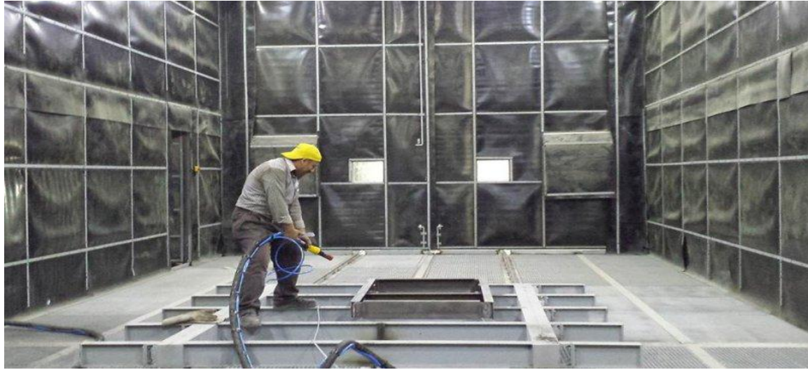
Manual blasting chambers
